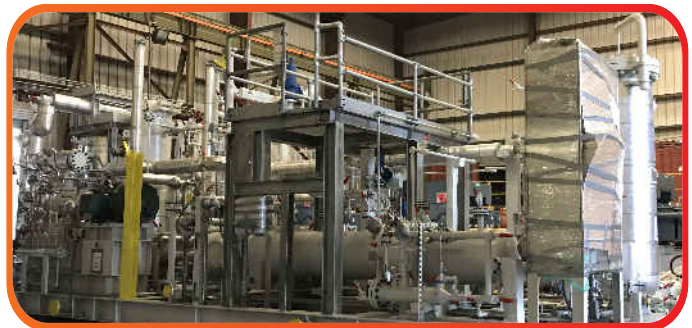
Process Refrigeration System
